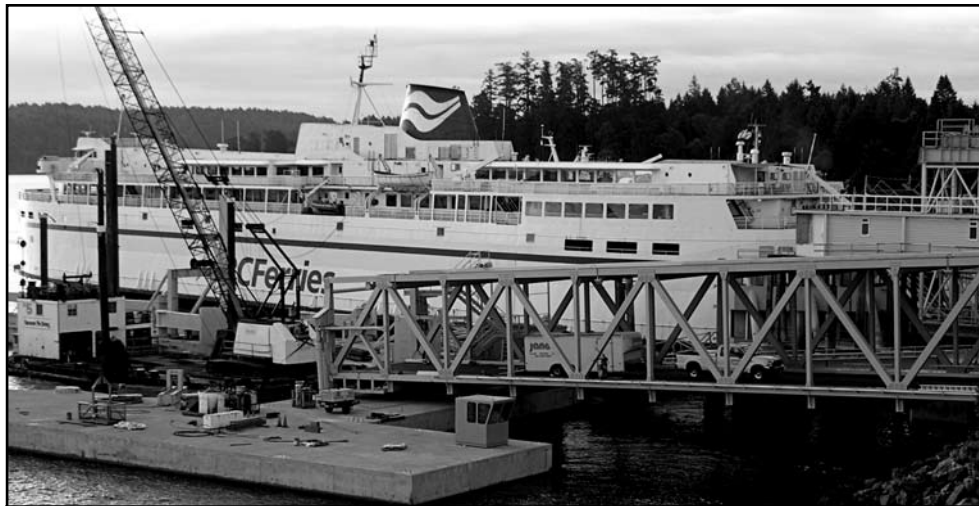
Emery Electric is doing the power and electro/hydraulic system on berth 2 preparation for the new Super “C” class ferries coming from Germany.
