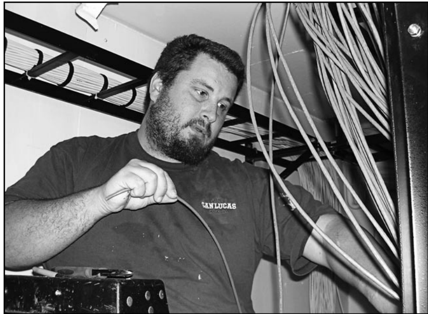
New Apprentice Christian Zarry helps sort out Data closet.
